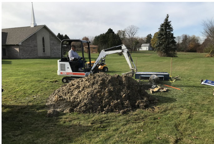
Elder Mike Shayna with his mini-excavator digging up the cement ball and sign post
