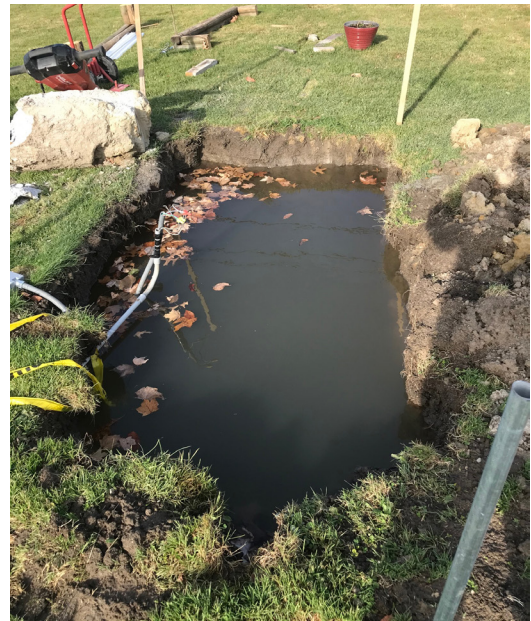
Water issues with church property uncovered by excavation for sign footing replacement
